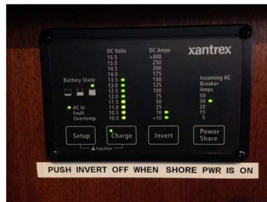
CLOSE UP VIEW OF THE INVERTER PANEL
