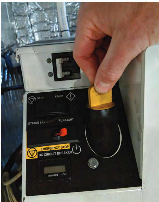
GenSet start at enclosure
