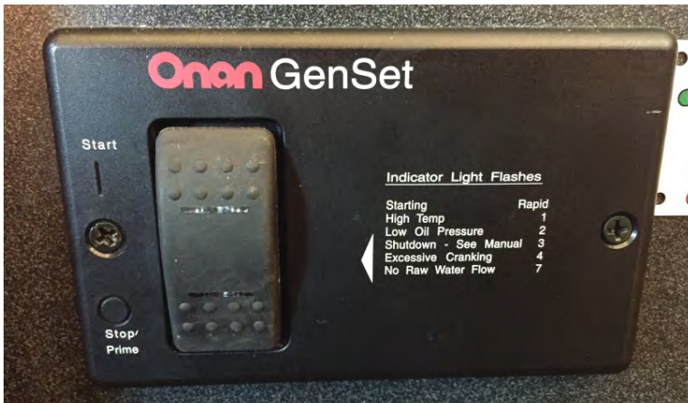
GenSet start at AC panel
