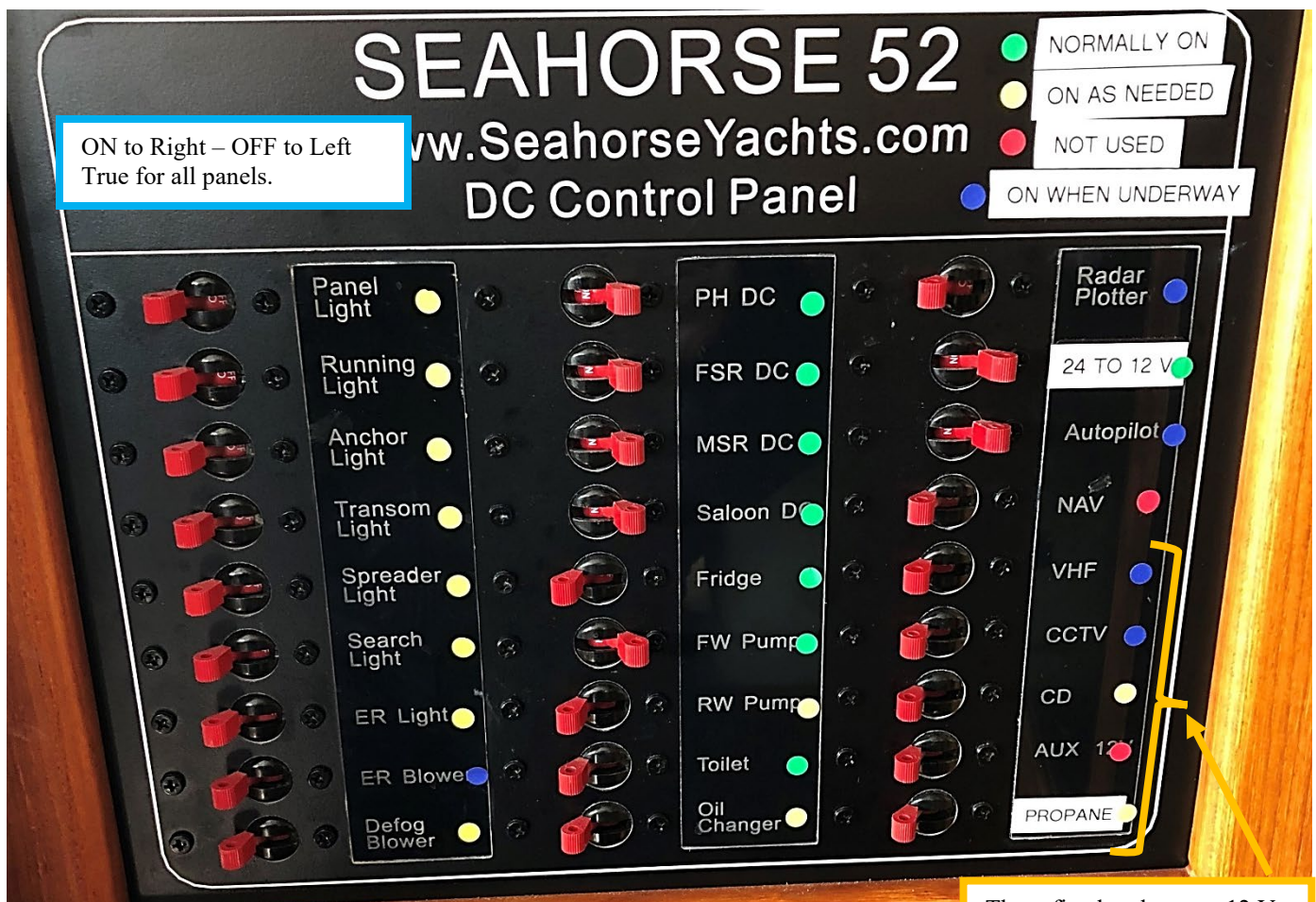
These five breakers are 12 V and need the 24 to 12 V breaker on to get power.
