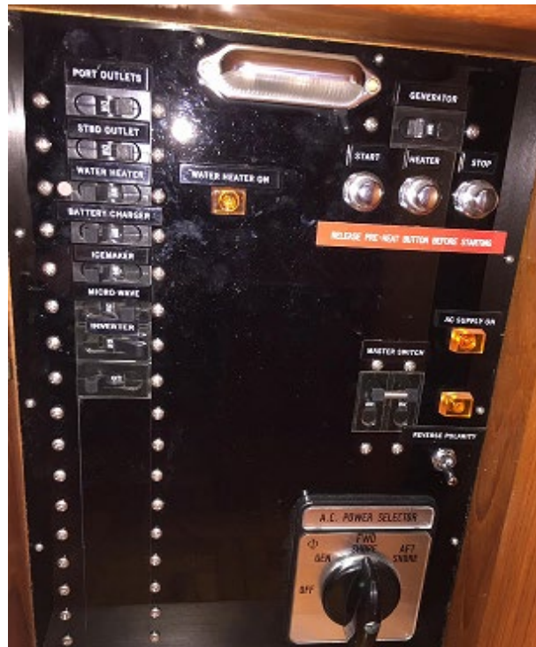
The AC panel controls 110-volt AC power throughout the vessel whether it is received from the shore power cord or generator or inverter.
