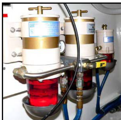
Starboard engine fuel filters mounted on side of starboard fuel tank. Two on left are switchable for the starboard main engine; filter on right is for the generator.
