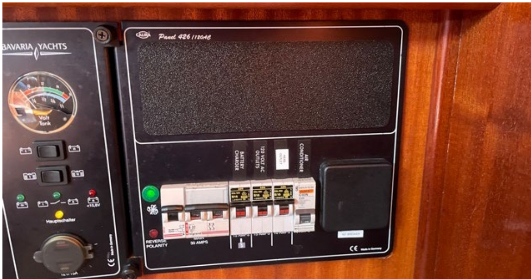
Turn on all 6 AC breakers when at shore power. UP IS ON (counterintuitively, you see the red part of the switch when it is turned on and the green part when it is turned off.)
