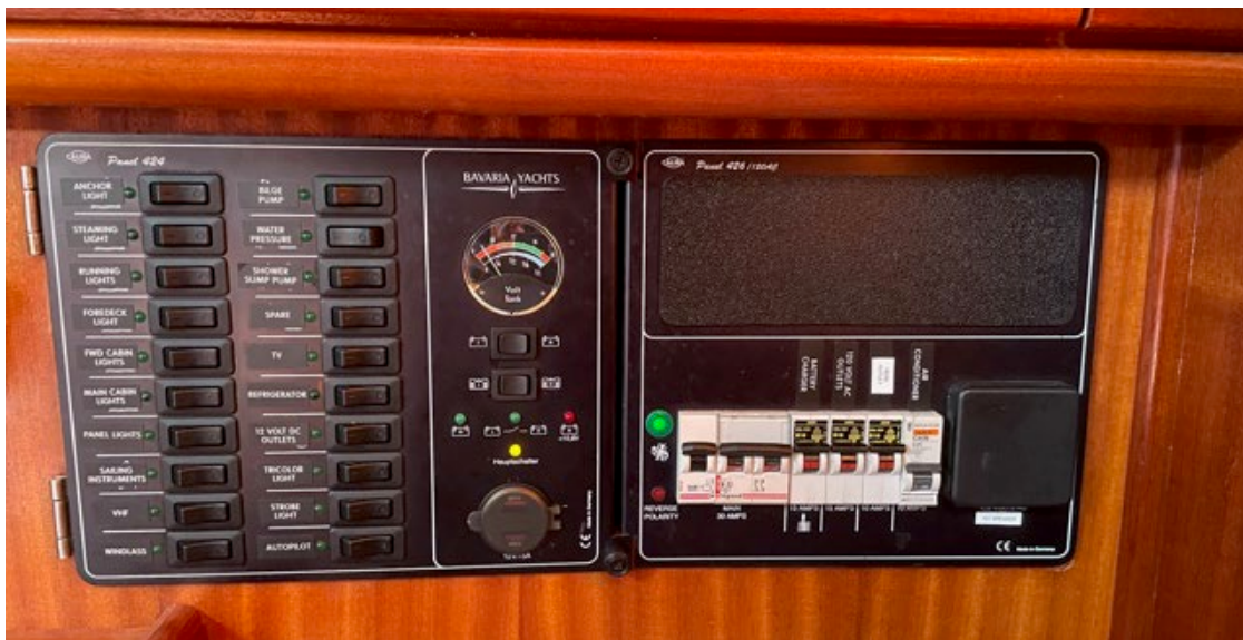
All breakers are located on the electrical panel, above the nav station. You will also find the voltmeter (used for the start battery only) and water tank gauges here.
