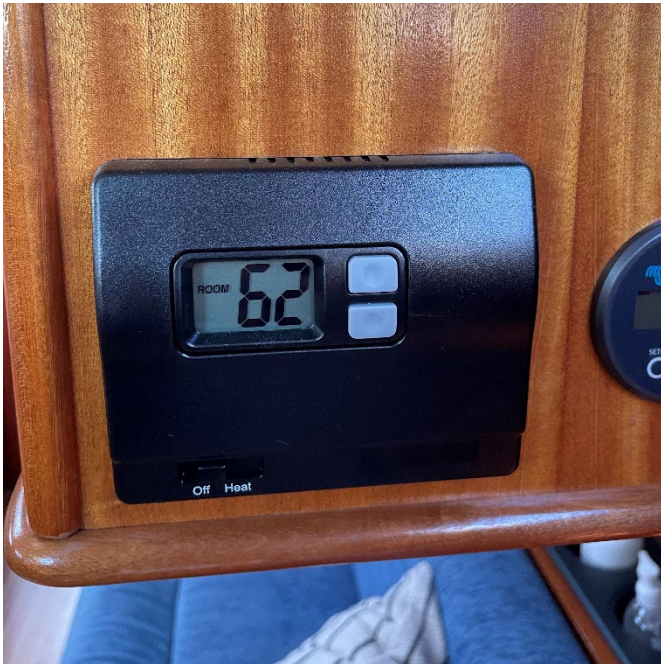
Furnace thermostat (okay to leave set to "heat"). Located above forward end of nav station.
