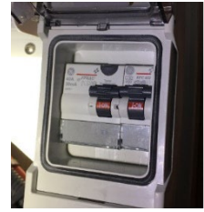
Primary Shore Power Breaker
