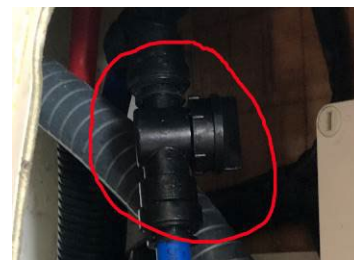
The photo above shows what the valve looks like. The valve is circled in red. The handle is on the right side in this photo.
