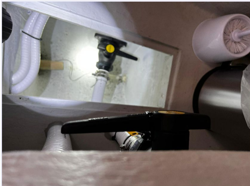
Starboard Holding Tank Lower Seacock Valve
