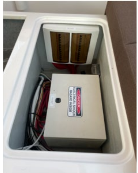
12V DC Breaker Panel
