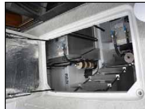
A look into the lazarette; the ladder eases engine room access.
