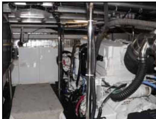
Forward to starboard, the other Cummins Diesel is right, the Onan genset is forward, and the bowthruster batteries are in the box aft of genset. The room is neat, brightly lit, clean.
