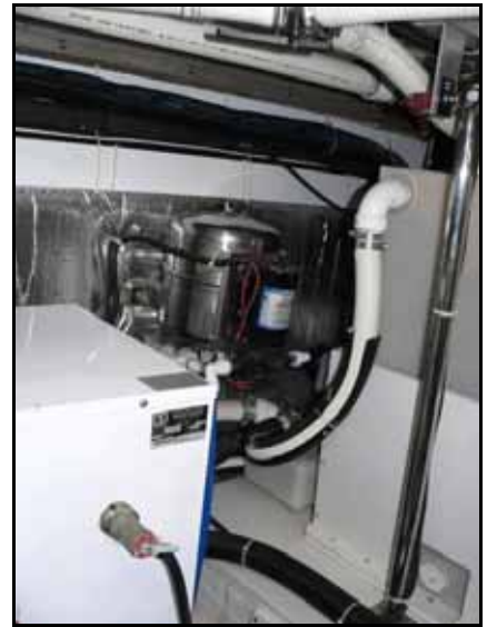
The water pump is in the engine room starboard side forward just to starboard of the hot water heater.
