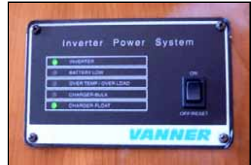
Inverter control panel by DC panel.
