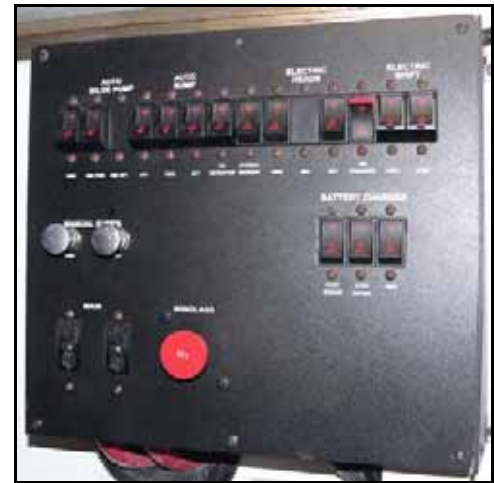
Engine Room DC Power Panel.
