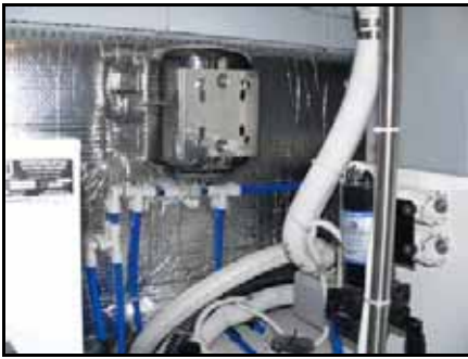
High in E/R forward starboard corner: Fresh water pump on right, corner of water heater left.
