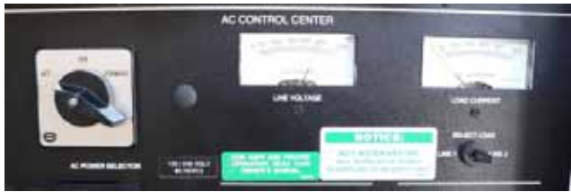
AC Panel, Metering & Power Selection section.
