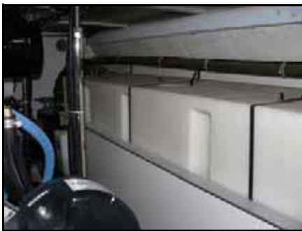
Port engine outboard: Water tanks and aft just past stainless support, port engine coolant tank. (Starboard is mirror.)
