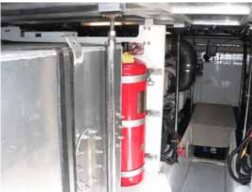
Looking forward to port from the lazarette the red engine room fire system is visible and past it the port engine.
