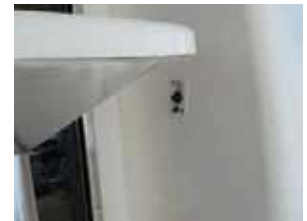
Light switch beside ladder to boat deck.
