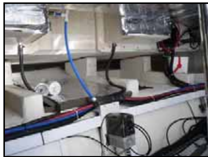
Aft center of lazarette: The trim tab pump is lower center, and piping for water and drains is apparent.
