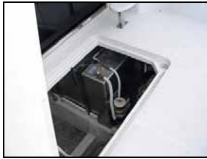
The hatch raised; the steps to the boat deck in the corner of the cockpit visible at top. (Another view of the ladder is on page 1.2) In this view you can see the fuel tank & starboard Racor.
