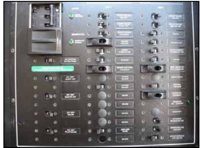
AC Power Panel, Switch section.
