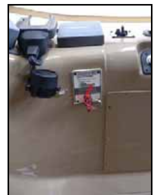
Engine Room Fire Extinguisher emergency control in the pilothouse: Pull pin and then pull handle to activate. See notes re the fire system in this manual...
