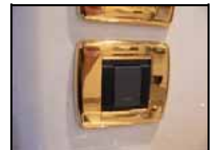
One of the head power switches. It carries the word "toilet". The top must be pushed in unless the head has failed!
