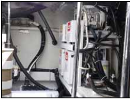
Laz starboard: Air conditioning controls with compressors behind and seawater pump below.
