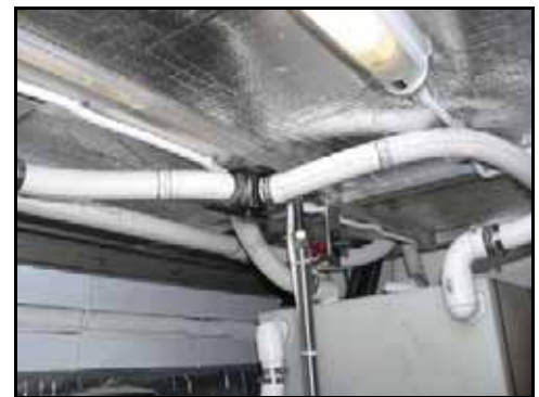
Y-Valve on ceiling of Engine Room port forward. Switch for overboard pump (red).
