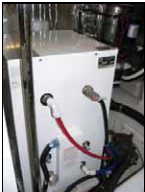
Water heater E/R forward.
