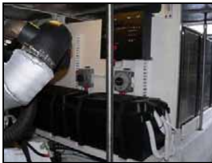
E/R stbd. aft: Exhaust pipe in foreground, batteries, battery switches for starboard engine & house, E/R DC panel above.
