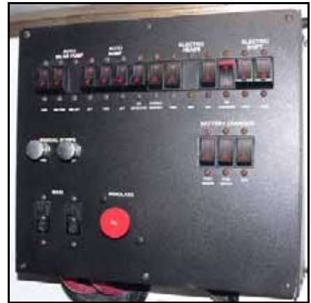
The E/R electric panel has breakers/switches for the bilge pumps, shower sumps, windlass, & battery chargers.
