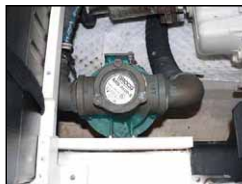
Port main engine sea strainer in foreground; its valve is just on the far side of shaft, with blue handle on far side “up”/open.
