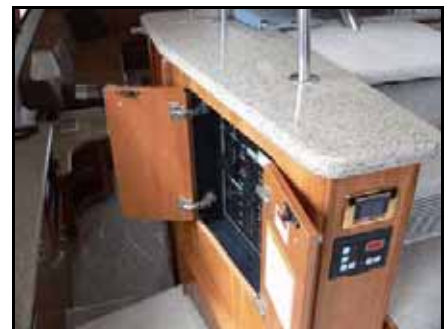
AC cabinet with door open. The DC cabinet is down the salon steps.
