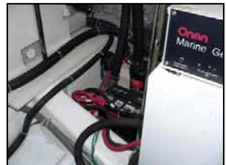
Down low, just port of the generator is its battery and, further to port, the port head's Vacu-Flush pump.
