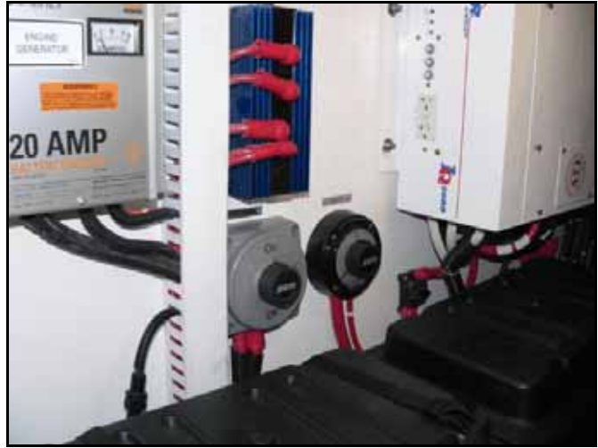
E/R aft port corner. 20-amp charger (left) is for the engine and generator batteries. Blue battery isolator. The large white box is the 2600-watt sine-wave inverter. Battery switches control port engine, davit.
