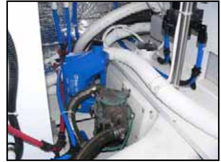
Low in forward starboard corner of engine room: Generator sea strainer, fresh water pump, spare oil. The Vacu-Flush pump for the starboard head is in lower right corner of photo.
