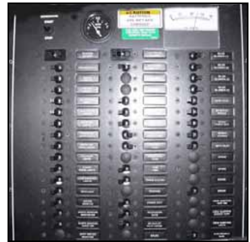
The DC electrical panel. At top is the fresh water gauge & house battery DC voltmeter.
