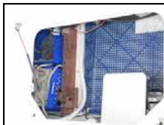
Inside the swim step center hatch.
