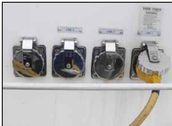
The shore power connectors are on the starboard side of the boat just aft of the side door. The left connector is for TV/phone, while the others are Line 1, 2, & 3.
