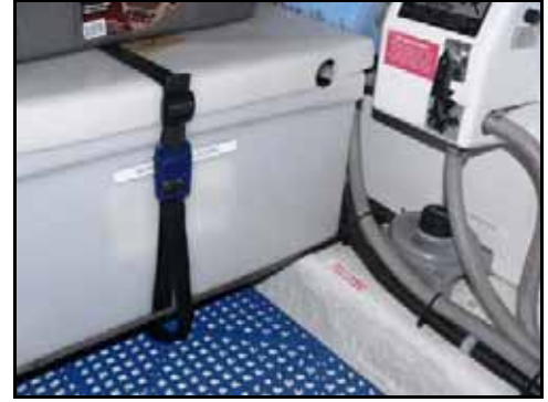
Here is one of the battery boxes (for the thrusters). This one is in the utility room under the hatch at the aft end of the companionway. Other batteries are in the lazarette.
