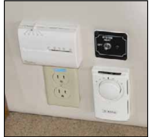
Just above the wet bar in the salon are the Diesel Furnace Thermostat and main switch (top) and an electric heater thermostat (bottom right).
