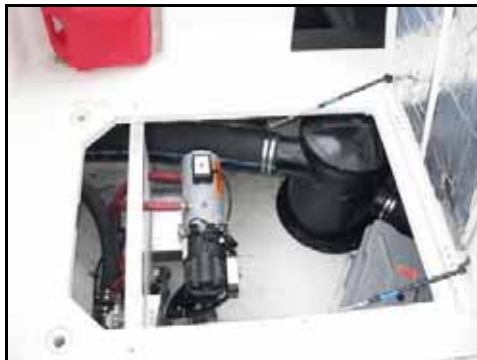
Under the port cockpit hatch is the lazarette with the Webasto Diesel furnace, the port engine muffler, and a (grey) battery box.
