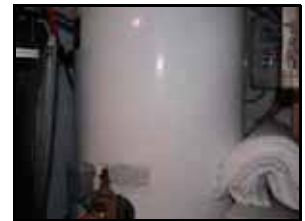
The water heater is hard to miss in the utility room!
