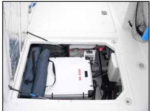
The Westerbeke generator under the middle cockpit hatch, with associated equipment and the stern thruster master switch. The folding chairs are atop the genset cabinet.
