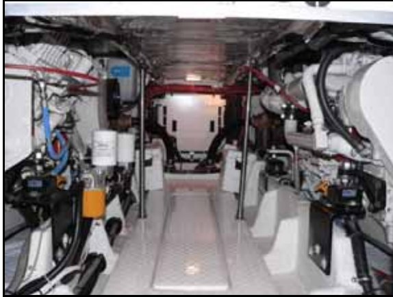
Looking aft through the utility compartment at the engine room. The Cummins engines are to each side, while the Westerbeke generator sound shield cabinet is all the way aft; right in front of the Westerbeke cabinet you can see the sea water hoses for the engines leading to the seacocks.
