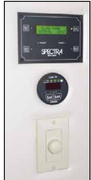
The watermaker control is in the pilothouse above the power panel. The Link 10 monitor and speaker control for nearby speakers are below it.
