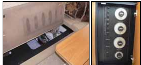
Some of the L-Settee's storage. Battery switches...
