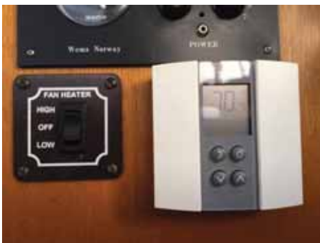
Thermostat and Fan Speed Control
