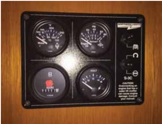
Generator Controller and Gauges
