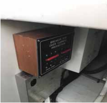
Aft: Lazarette Main House breaker
