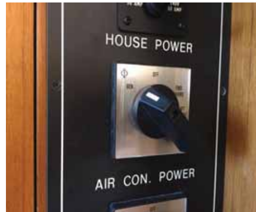
House Power Generator Switch
