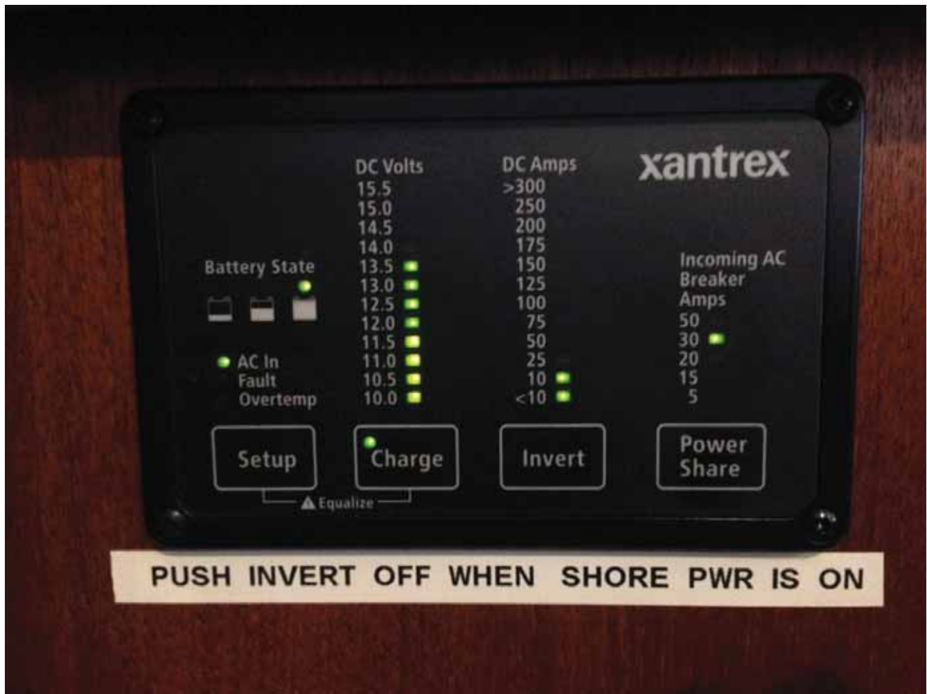
CLOSE UP VIEW OF THE INVERTER PANEL
