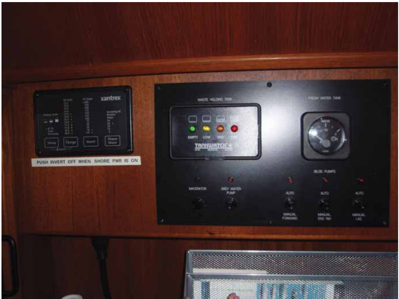
XANTREX INVERTER PANEL and TANK WATCH PANEL
