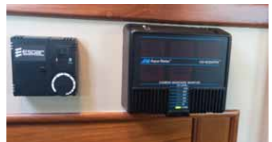
Espar Diesel Furnace Control and Carbon Monoxide Monitor
