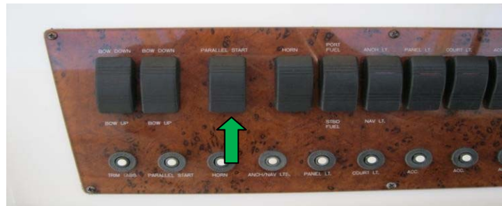
Battery Parallel Start Switch
