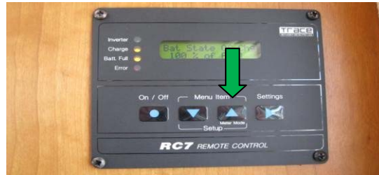
Inverter Control Panel and Meter Mode Switch
