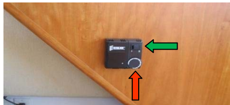
Diesel Heater Control _ Temperature and On/Off
