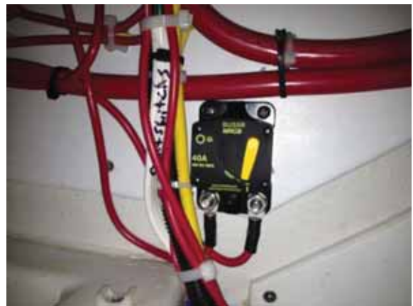
Davit Control Circuit Breaker
