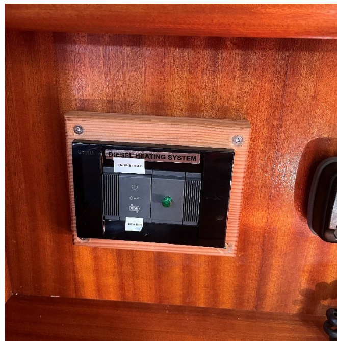
Main on/off switch for furnace. Located above outboard side of nav station.
