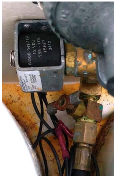
Figure 1 Small valve below solenoid in propane locker.
