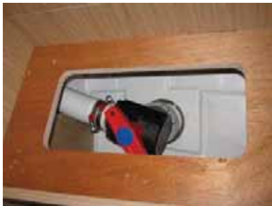
Aft Head Overboard Discharge Valve – Located in Starboard Cabin under Access Panel in Front of Hanging Locker
