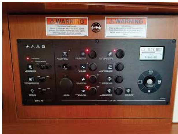
Electrical Panel – AC Controls on the Left, DC controls in the Middle; Toggle Switch and LED on the Right are used for Checking Battery Charge and Tank Levels (Fuel, Water)
