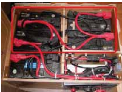
Battery Bank – Aft Port Cabin
