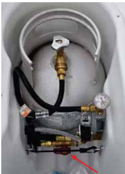
Propane Tank with Master Valve (top) and Red BBQ Valve (red arrow – valve in open position)
