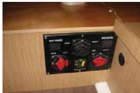
Battery Switches – Aft Port Cabin
