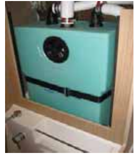
Black Water Holding Tanks
