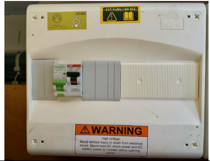
Aft cabinet AC Ground Fault Breaker
