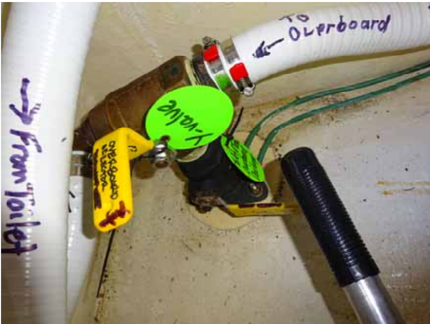
Tank to Overboard (Bent Handle Y-Valve and Seacock)
